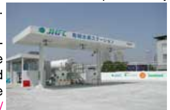
Shell Hydrogen Station in Tokyo
