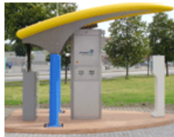
Stuart's Malmö Hydrogen Station
