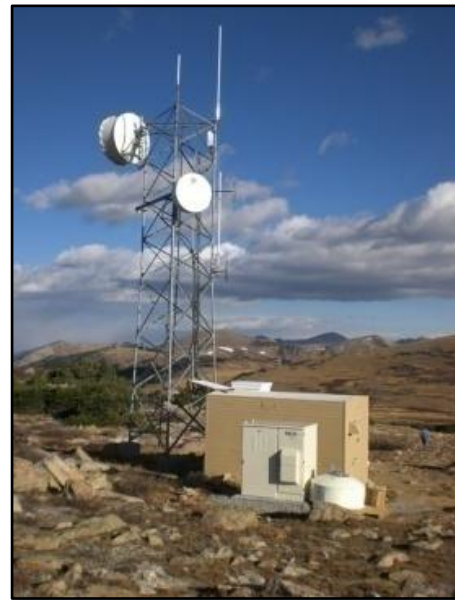
ReliOn fuel cell powering cell site
