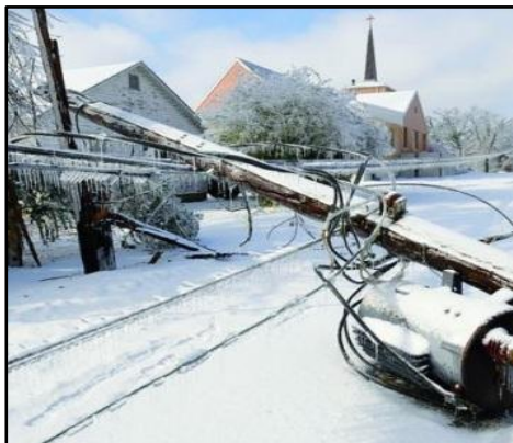
A downed power line in a snowstorm
