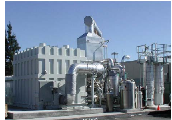
FuelCell Energy 1.4 MW system
