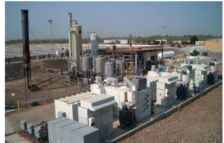
FuelCell Energy 1.2 MW system
